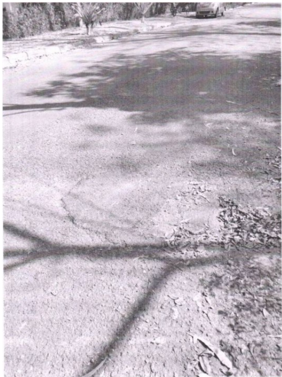
Figure 9: Fig: Cracked asphalt with potholes in main road residence area lane 32
