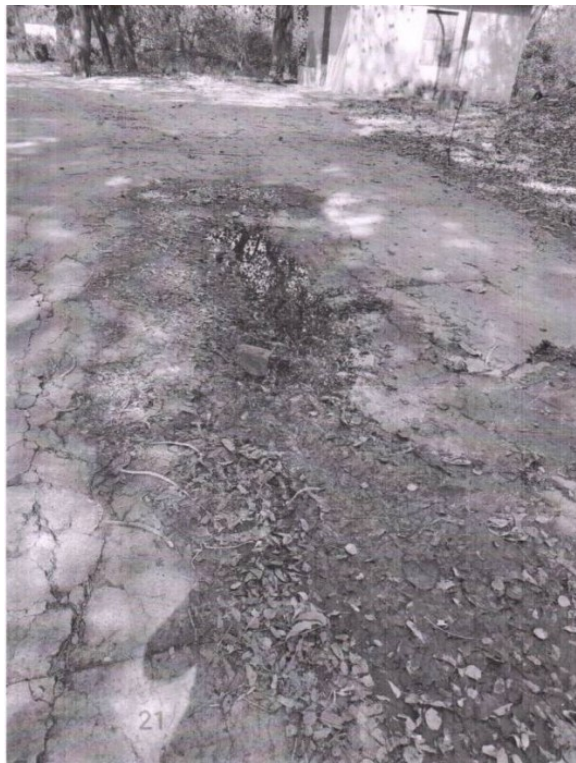
Figure 20: Fig: Cracked asphalt with potholes and stains in main road residence area lane 36
