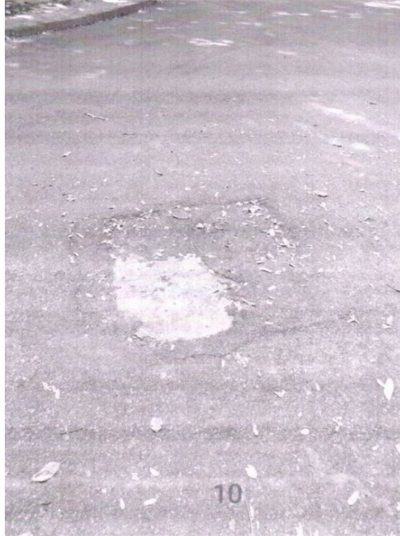
Figure 10: Fig: Deterioration of asphalt pavement in main road residence area lane 33
