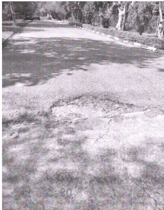
Figure 19: Fig: Asphalt road with large holes in main road residence area lane 36
