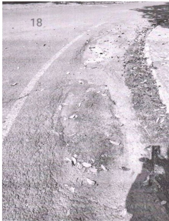
Figure 17: Fig: Cracked asphalt with potholes and stains in main road residence area lane 36
