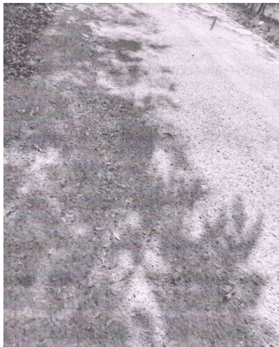
Figure 7: Fig: Deterioration of asphalt pavement in main road residence area lane 31
