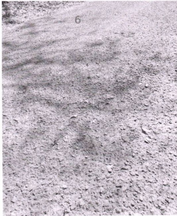
Figure 6: Fig: Cracked asphalt with potholes and stains in main road residence area lane 31
