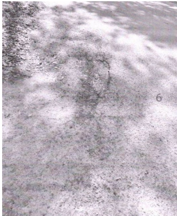
Figure 5: Fig: Cracked asphalt with potholes in main road residence area lane 31
