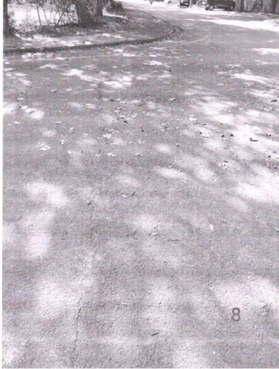
Figure 8: Fig: Cracked road surface in main road residence area lane 32
