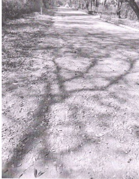
Figure 14: Fig: Deterioration of asphalt pavement in main road residence area lane 33
