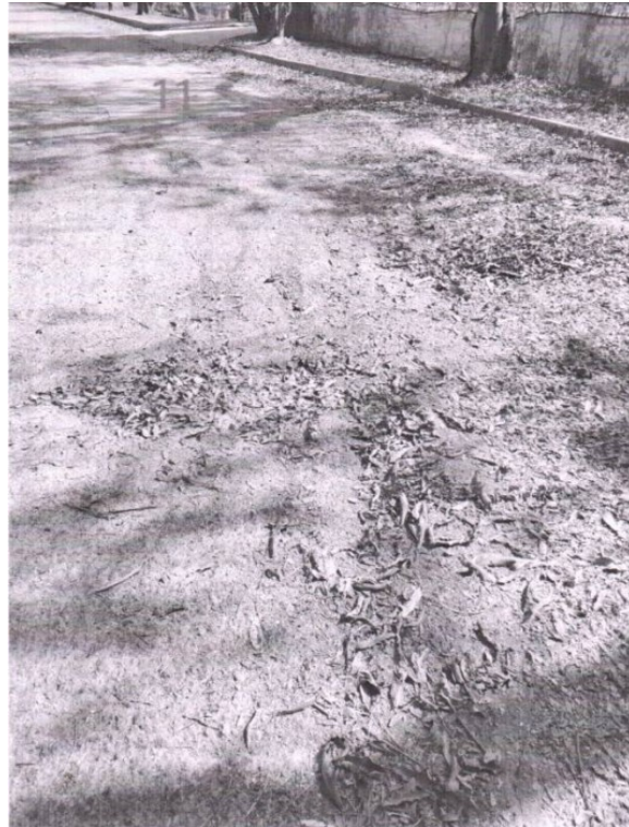
Figure 11: Fig: Potholes in main road residence area lane 33
