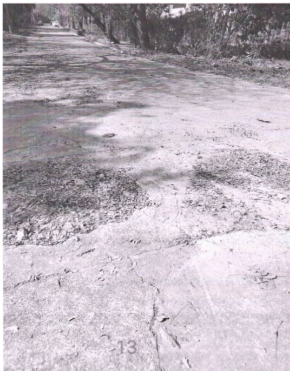
Figure 13: Fig: Damaged asphalt road in main road residence area lane 33
