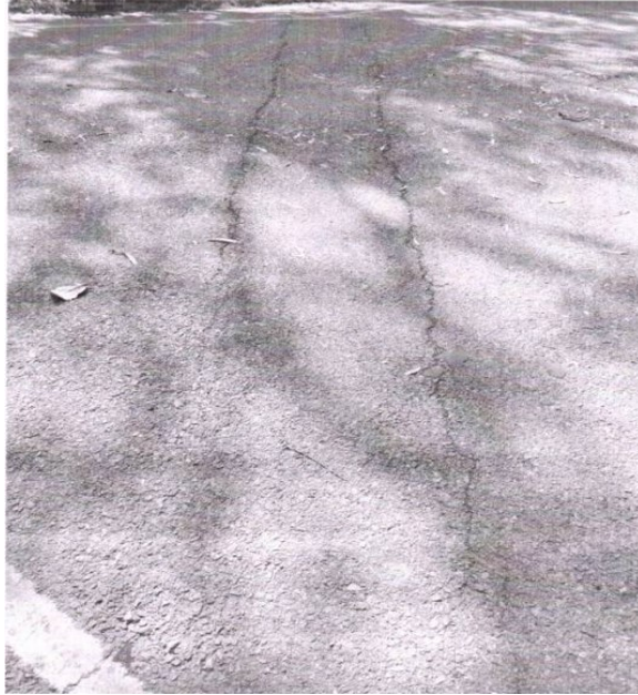
Figure 3: Fig: Potholes and cracks in concrete road in main road residence area lane 31
