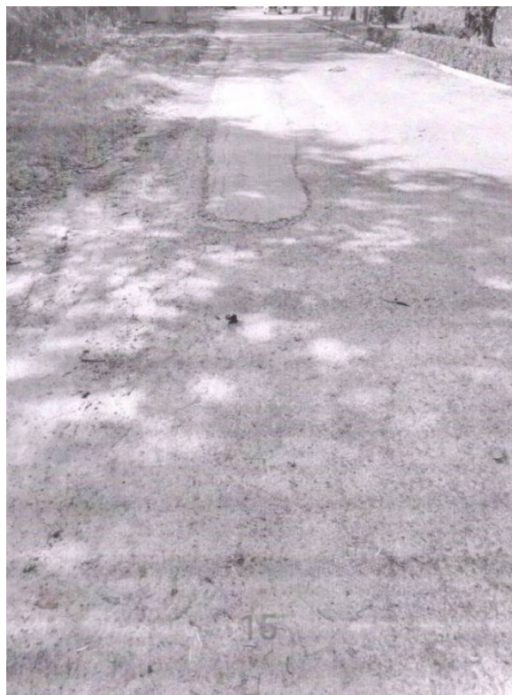
Figure 15: Fig: Damaged asphalt road in main road residence area lane 33
