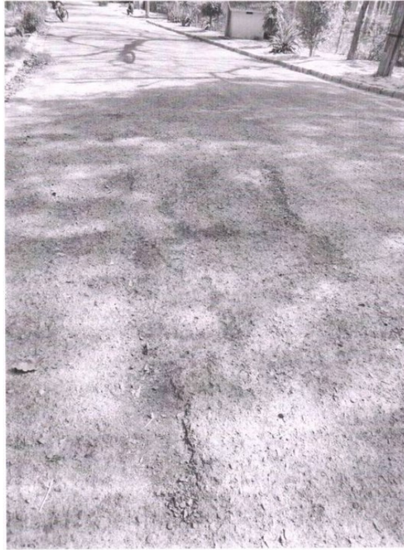
Figure 4: Fig: Potholes in road surface
